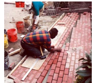
1992 Lombard Street San Francisco, CA, USA Repaving of one of the world's most recognizable roads
